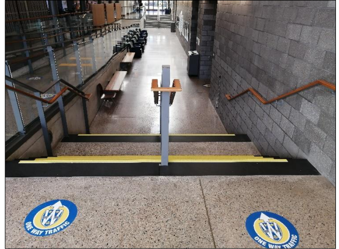
Colour-contrast stair stripping and tactile surfaces at ramp (left), Health Education Centre
