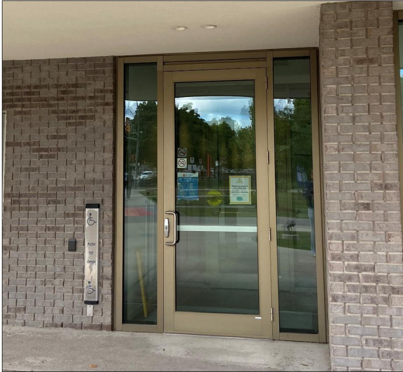
Accessible east entrance – ground level with actuators
