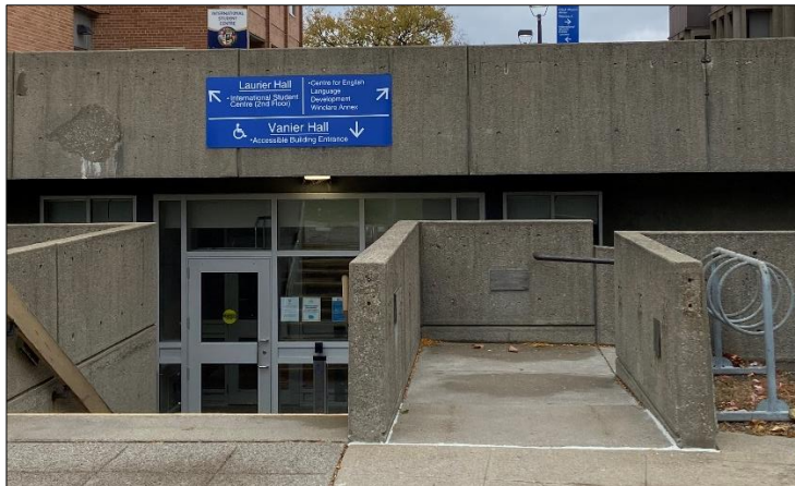
Ramp is located on the right and leads to actuator-operated doors on the north entrance.
