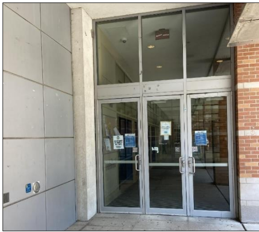
Outside the main entrance at CAW Student Centre. Ground-level with an actuator.
